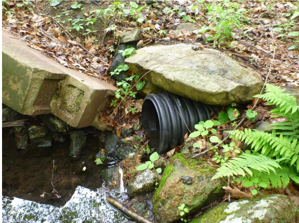
May 2016 photos of inlet to Mamanasco Lake
